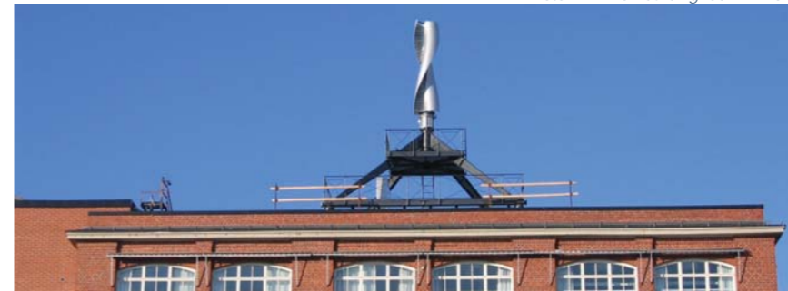
Photo: HAWT on building roof in Finland
