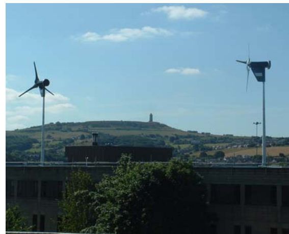
Two 6kW wind turbines installed in May 2006
