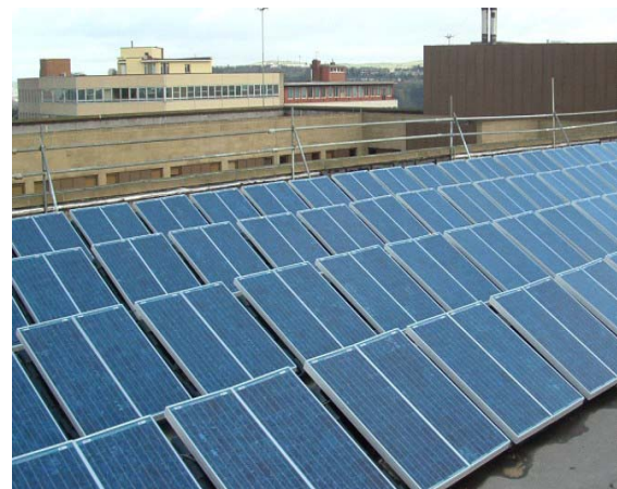
17.6kWp Solar PV installed in February 2005
