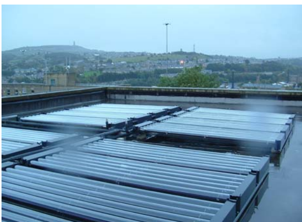
48m 2 solar thermal systems installed in February 2005
