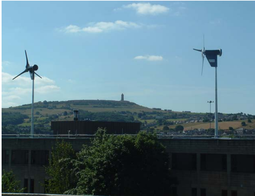
Two 6kW wind turbines installed in May 2006
