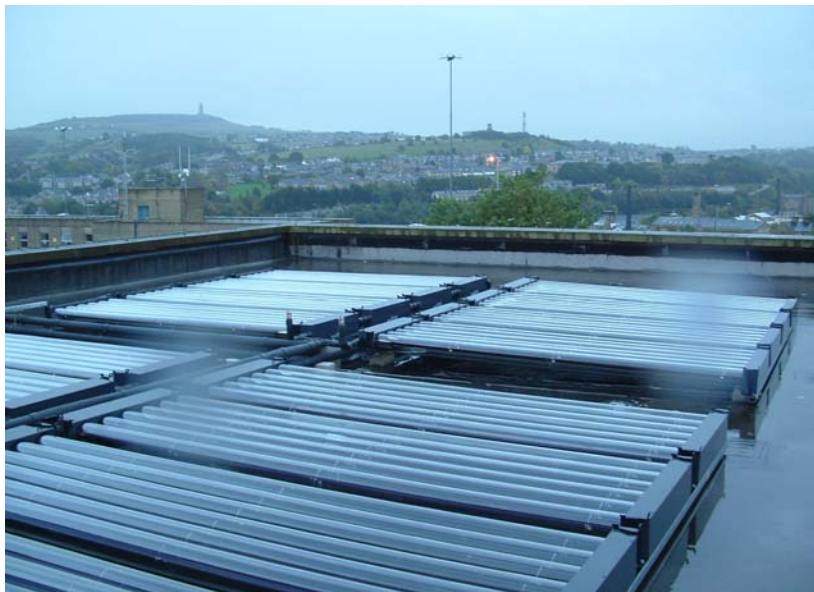
48m2 solar thermal systems installed in February 2005
