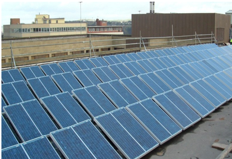
17.6kWp Solar PV installed in February 2005
