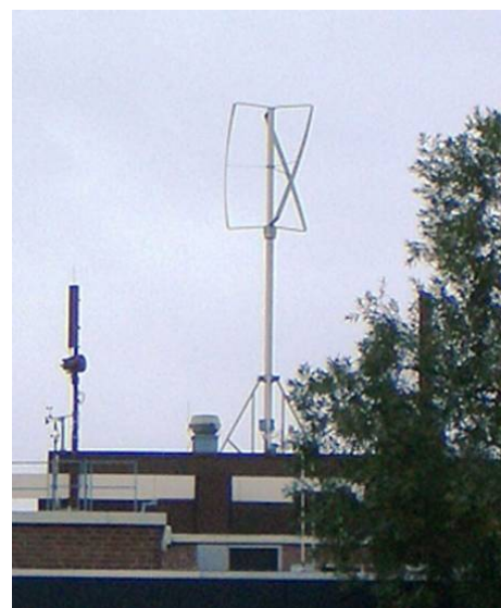
Figure 1: Turby, small wind turbine on a public building, Hoofddorp
